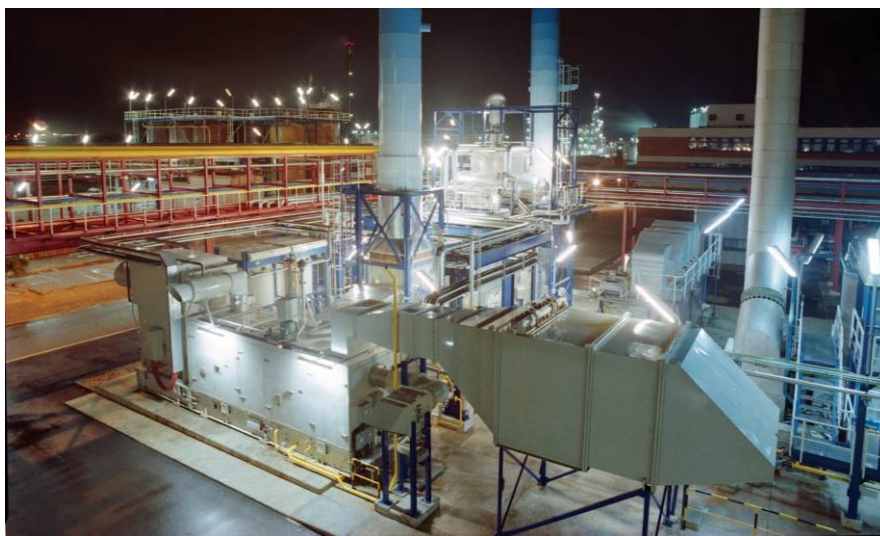
Figure 3: SGT-200 unit operating on high-hydrogen fuel at an oil refinery in the U.K.
