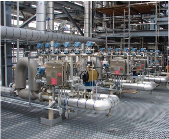
Figure 5. Fuel blending system installation at launch customer site.
