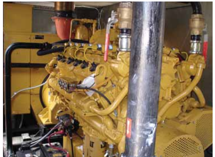
The three-phase, 405-kilowatt Caterpillar generators are rated at 506 kilovolt-amperes, 480 volts, 1,800 revolutions per minute, and 60 Hertz.
